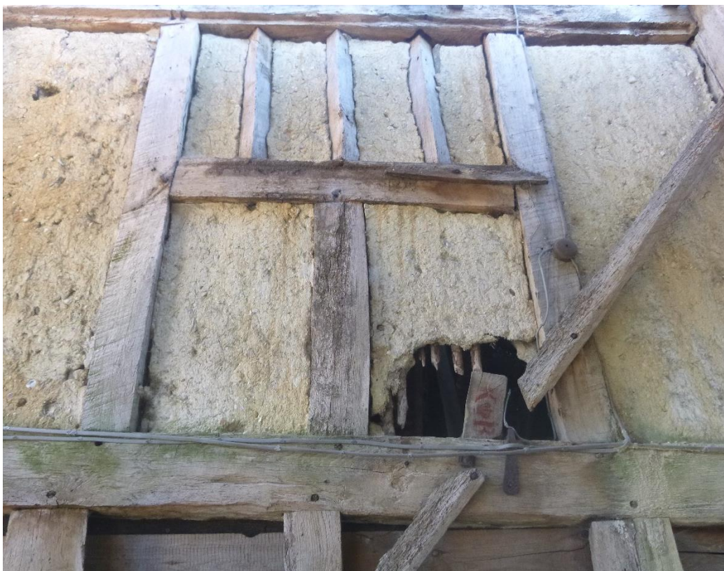
The eastern-most first floor window, internal view, showing the diamond mullions and the form of wattle and daub infilling
