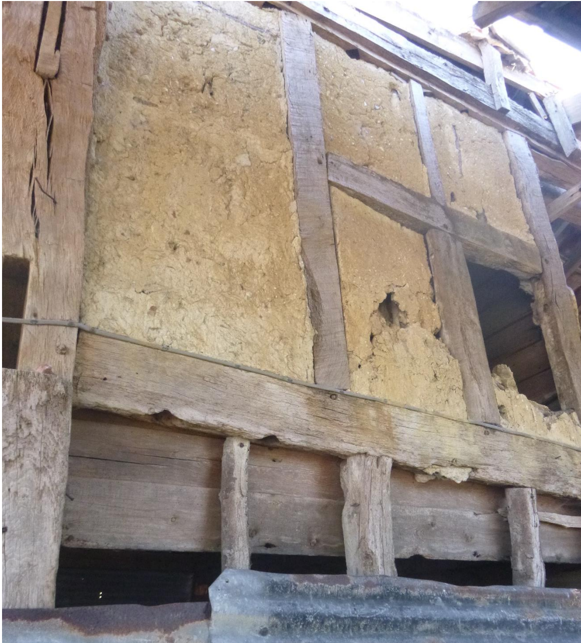
The central first floor window (infilled) with the joints for a ground-floor window visible on the underside of the girding beam. The wall plate is above the first-floor window and the easternmost surviving truss post of the south wall to the left
