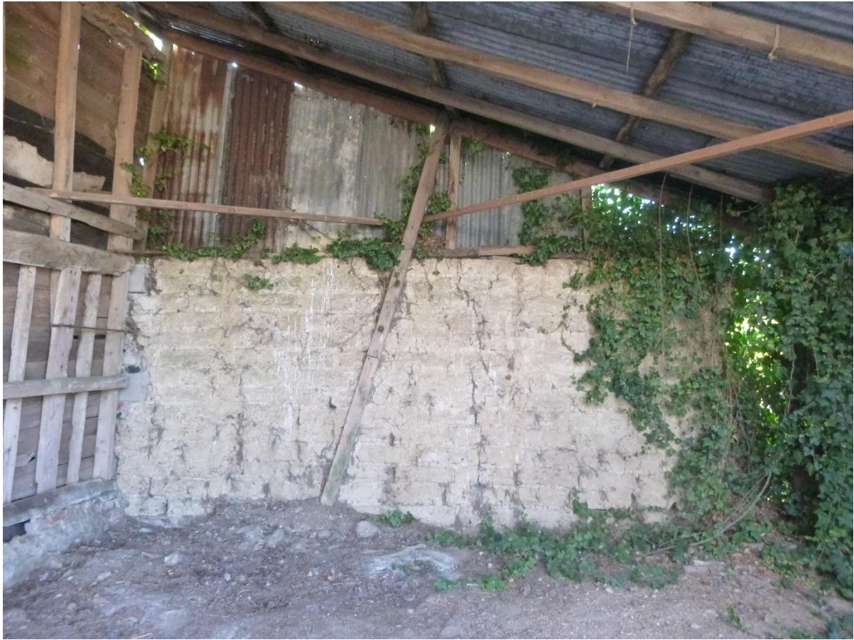
The western gable, completely replaced by a c.19 th century clay lump wall and 20 th century corrugated iron.
