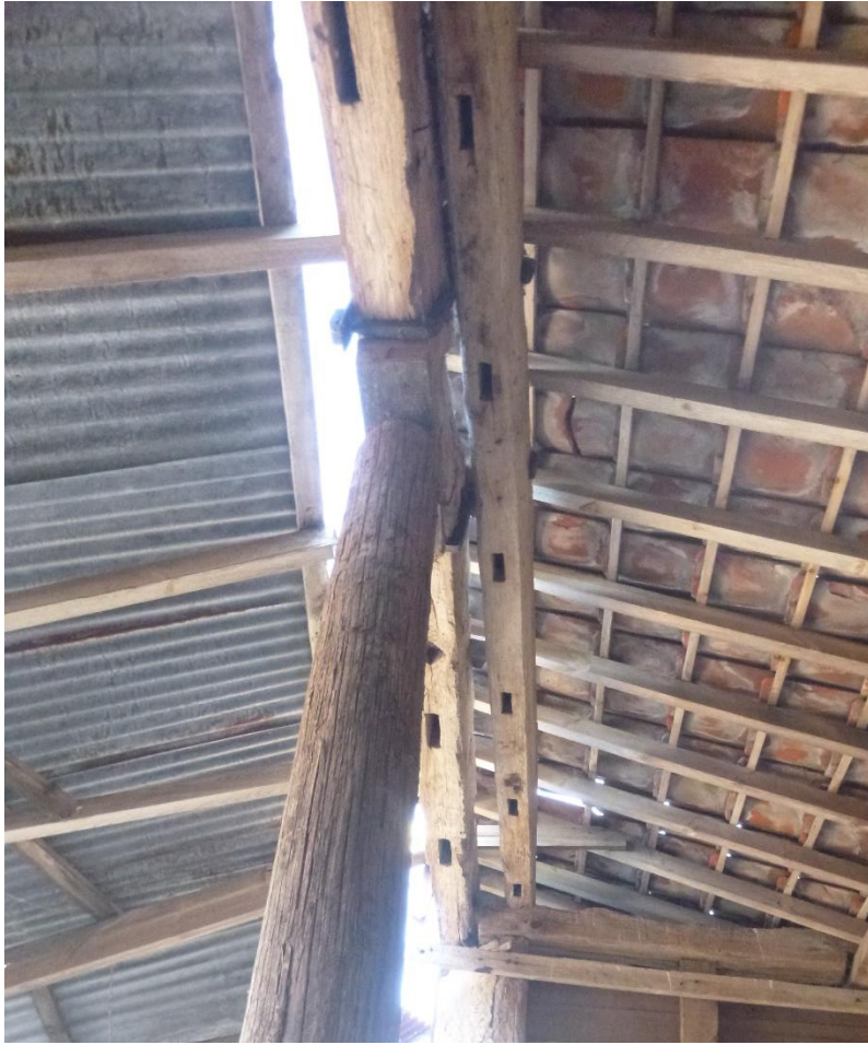
The failed wall beam by the 19 th century south doorway. The 19 th century barn porch is to the right, the central cell of the 17 th century house to the left. The joints on the underside of the wall plate are for the wall studs, and one window mullion is just visible behind the telegraph post. The telegraph post supports the failed scarf joint, which had previously been strengthened by the addition of a reused 17 th century beam (probably an unneeded girding beam) joined to it by iron framing.
