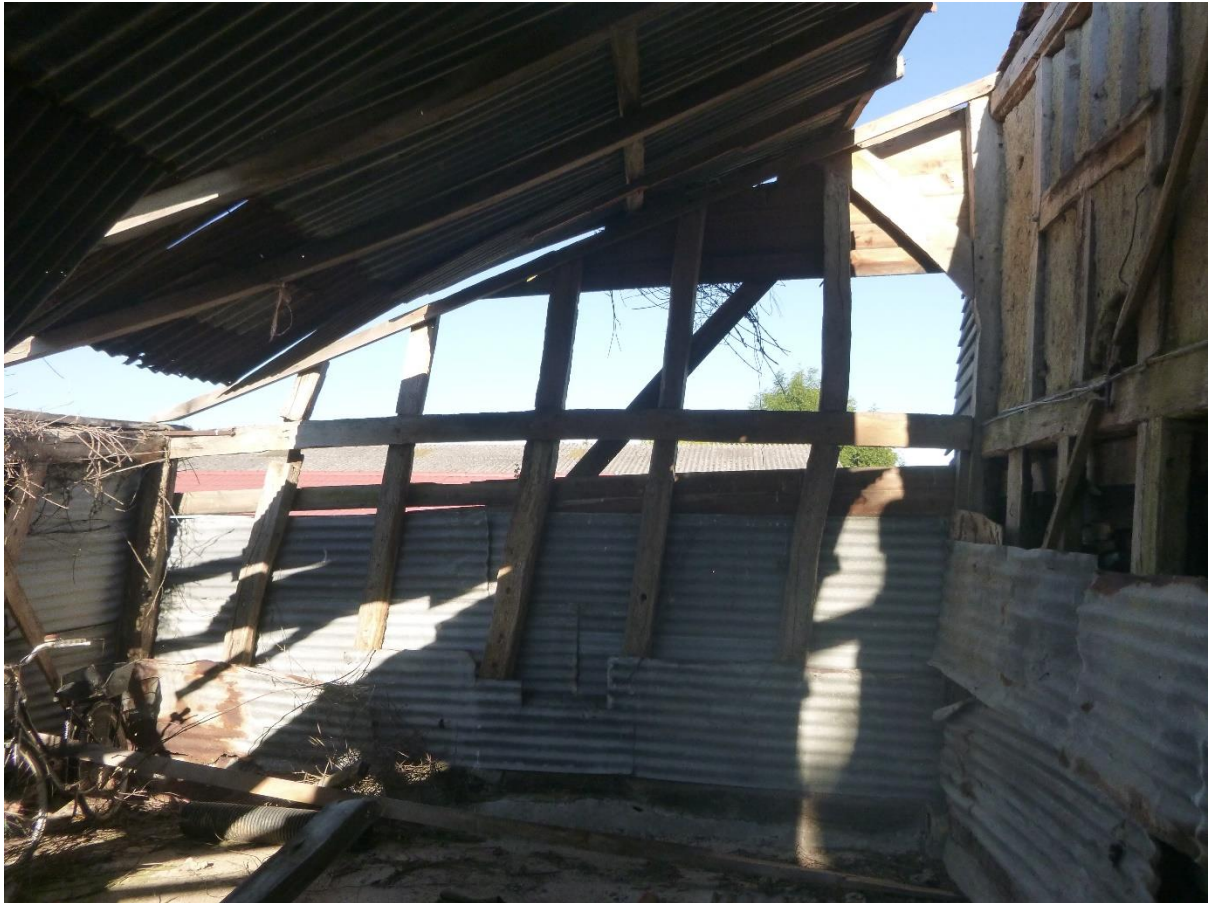
The eastern gable with a girthing beam (the horizontal beam) and one surviving brace (the upper right diagonal beam) and some original wall studs (the smaller, vertical beams)
